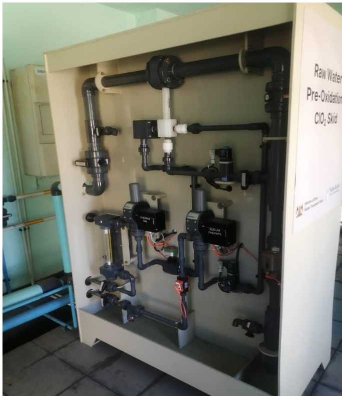
Chlorine Dioxide dosing point on the clarifiers
