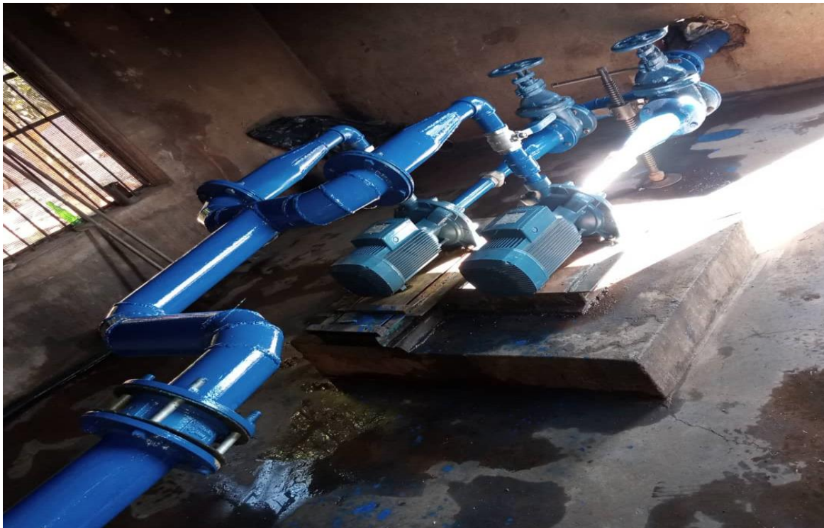
Newly installed pump sets and valves at Arcturus Road Pump Station
