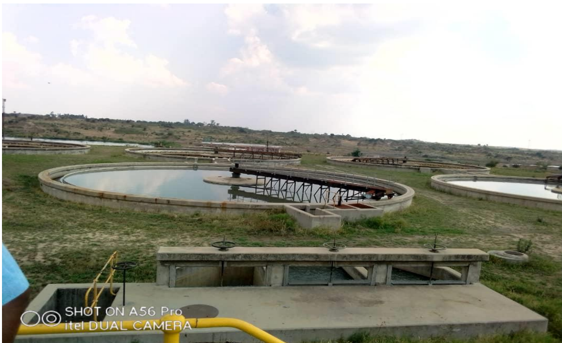
Newly commissioned Firle Unit 5C Clarifier
